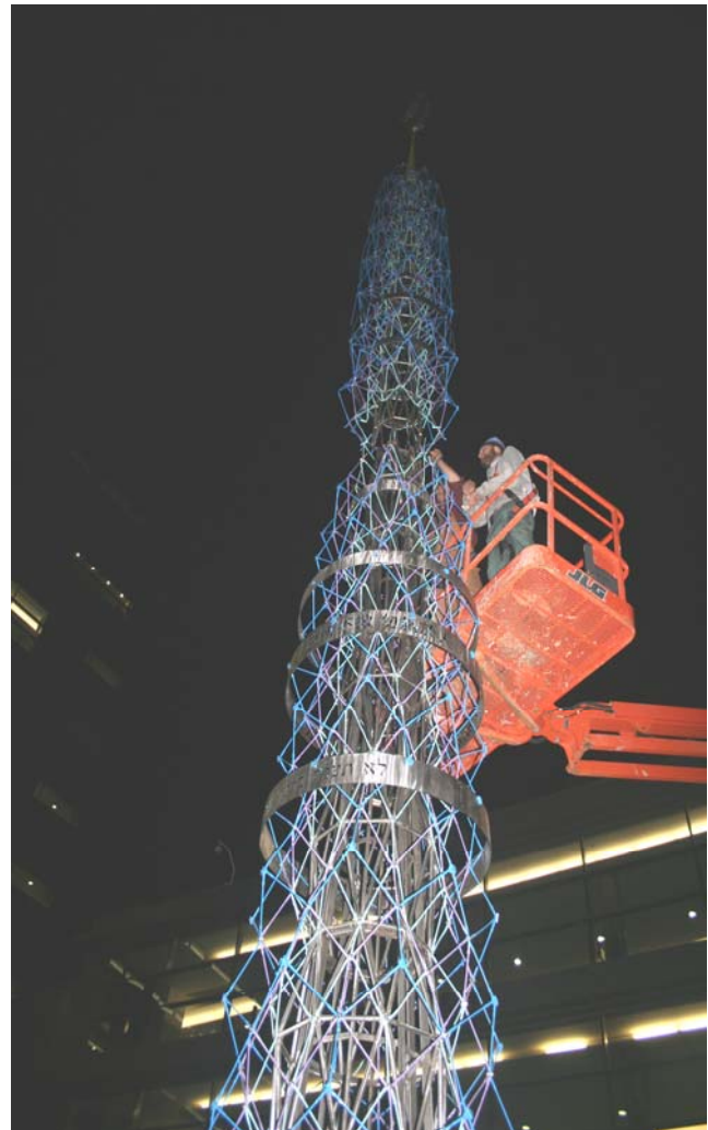
The Brower Hatcher sculpture under construction on the New Castle County Courthouse Plaza—November 13-17, 2006
