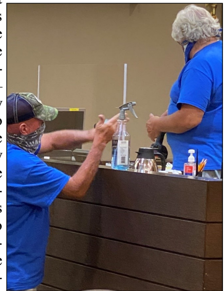
Work crews installing clear plastic shields in a Wilmington courtroom in June 2020.
