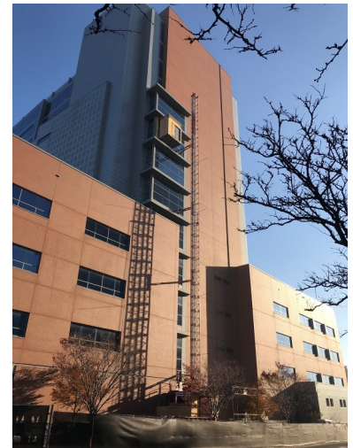
LEFT: An air handling unit is moved into place, via crane, to the 7th floor of the LLWJC in April 2020. RIGHT: From November 2019, a construction elevator installed on the outside of the LLWJC to carry materials to the 7th floor.
